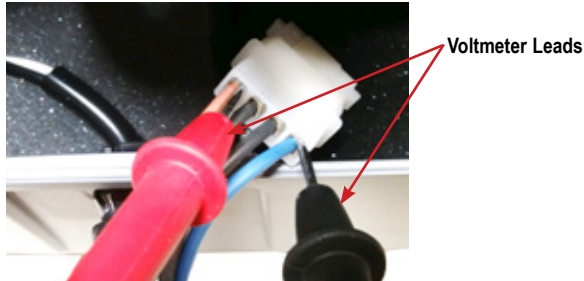
Testing Compressor Voltage
